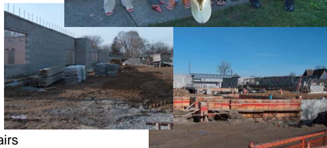
Photo collage: (Top) Vice Chair of the Board Linda Ward and Trustee Michelle Parks (centre) pose with principals of the four south Sarnia elementary schools at the official groundbreaking. (Below) Construction is underway at the Bright Street and Oak Avenue sites.
